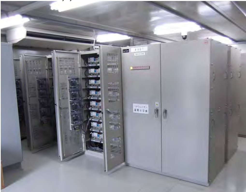
2. Lithium-ion battery system
